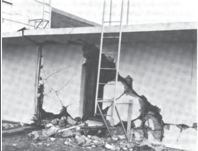
Close up view of pounding damage to the expansion joint between second floor of classroom wing and upper part of gymnasium. (National Academy of Sciences, 1973)
