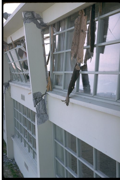
Close up view of damage to the column and beam joints at the second level of the classroom wing. (Comartin et al., 2004)
