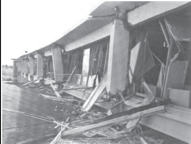
Close up view of second story columns and window sash, taken from the roof of the library. (National Academy of Sciences, 1973)
