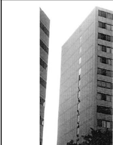
Classic shear failure of the coupling beams between linked shear walls at the south end of the building. (EEFIT, 1994)
