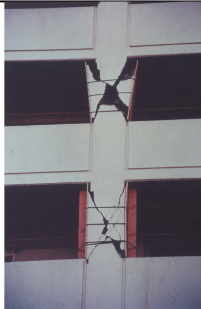
Typical X-shaped shear cracking, a result of induced short-column effects from the presence of balcony parapets. (Comartin et al., 2004)
