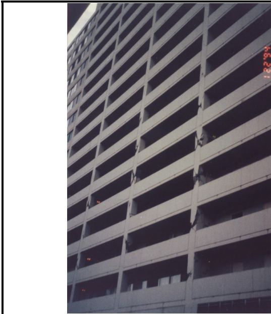
Damage to the perimeter moment frames of the Champagne Tower. (Comartin et al., 2004)
