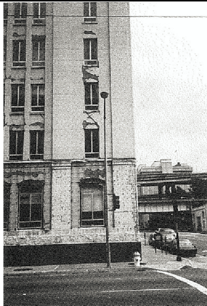
Cracking in exterior spandrels. (Schmid, 1991)
