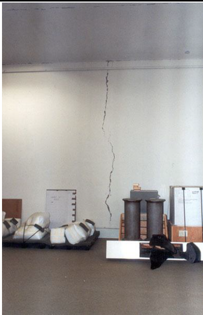
Damage to the interior of the museum. (Poland, 2006)
