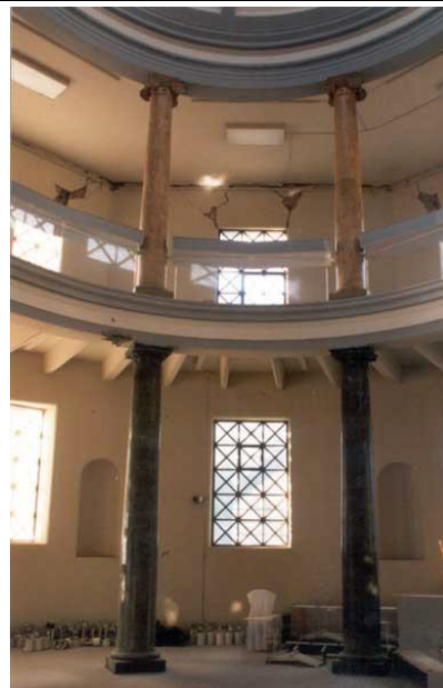
Damage to the interior of one of the octagonal rotundas. (Poland, 2006)
