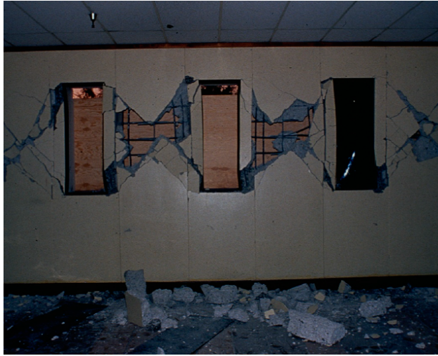
Damaged concrete shear wall at west wall, first floor. (EERI, 1994)
