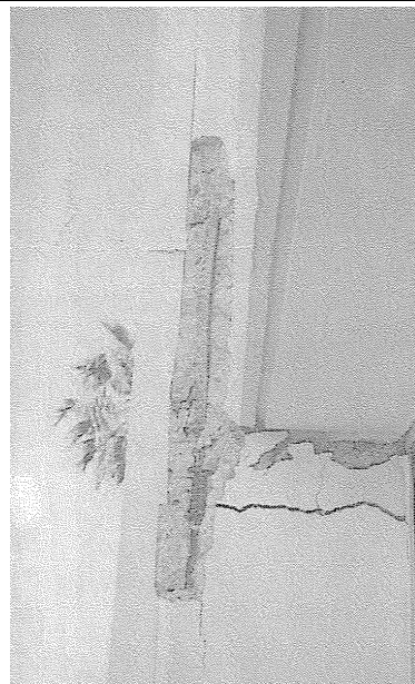
Close-up view of damaged exterior spandrel beam-column connection at fifth floor level. (SSC, 1994)
