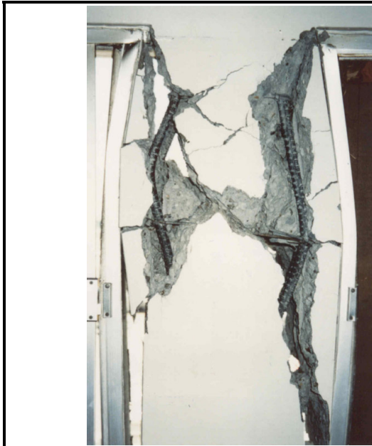
Close-up of x-cracking in column where tie failed. (Comartin et al., 2004)
