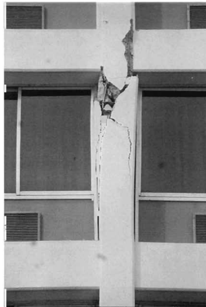
Close-up of x-cracking in column. (EEFIT, 1994)
