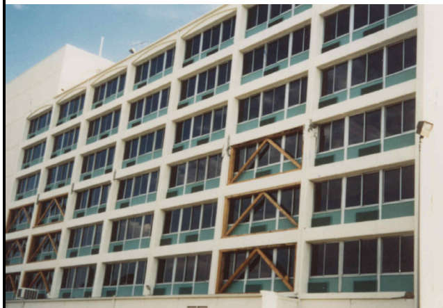
North elevation of the damaged building with temporary shoring in place. (Comartin et al., 2004)
