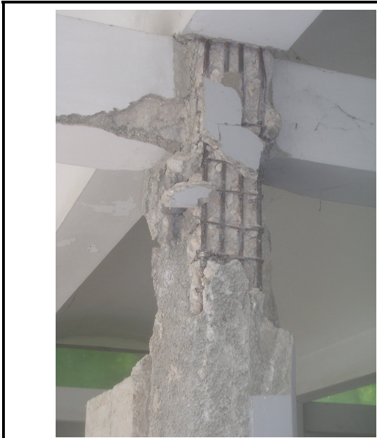
Shear damage to column and beam-column joint. (Federico, 2010)
