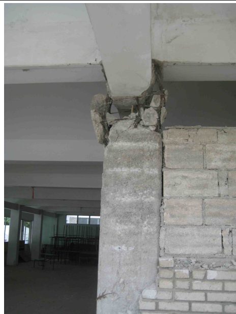
Severe shear failure in column adjacent to partial height URM infill wall. (Federico, 2010)
