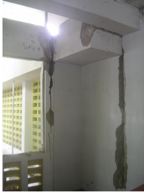
Shear damage to framing and URM wall from pounding between wings. (Federico, 2010)
