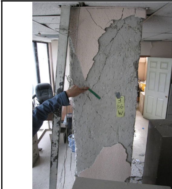
Shear cracking in column. (Telleen, 2010)
