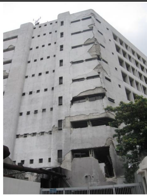
Damage to exterior of building. (Telleen, 2010)
